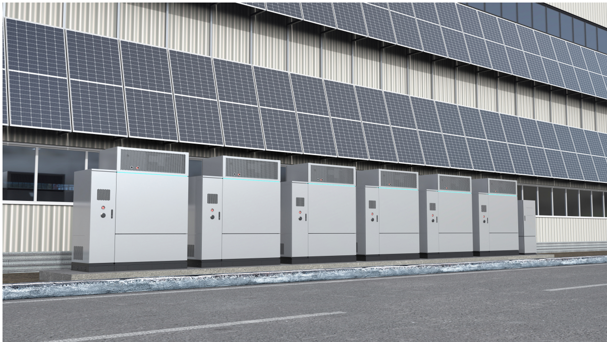
Multi-unit GridOne installation integrated with rooftop solar, a scalable energy storage solution for commercial and industrial sites.
